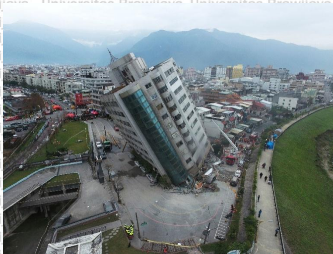
Figure 1. 1A large building damage on its first floor due to an earthquake in Hualien City (New York Times).
