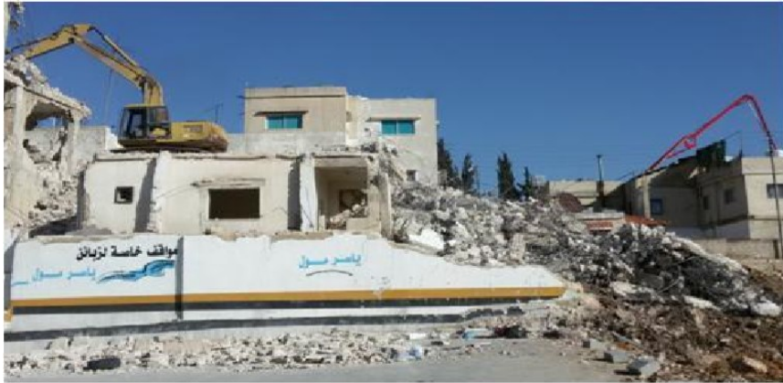
Figure 1.2: Building rubble in Jordan (Qasrawi, 2017)
