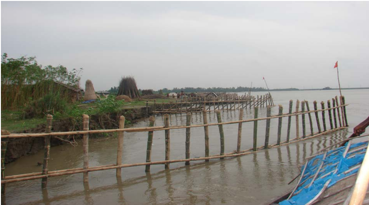
Fig.1. Bandalling construction work were going on in the Jamuna River of Bangladesh
