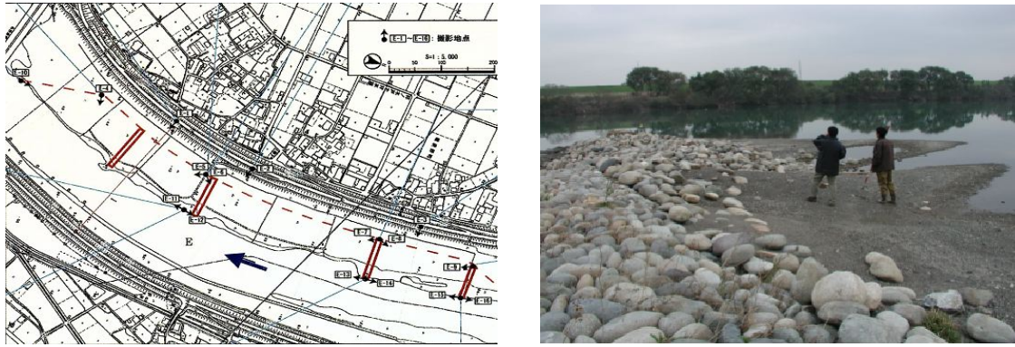
Figure 1 Groynes in compound open channel of the Ibi River, Ohgaki city in Japan (Left: Excavating work in the Ibi River, Right: Groyne and downstream sediment)
