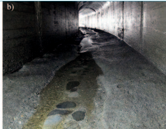
Figure 2. (a) Schematic view of an in-stream reservoir with sediment bypassing [7] and (b) abraded concrete invert of the Runcahez SBT, Switzerland (Photograph: M. Müller-Hagmann, VAW, ETH Zurich)
