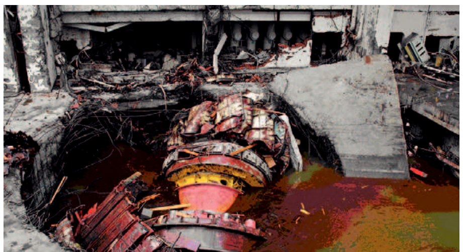
Figure 5. Unit 2 several hours after failure.
