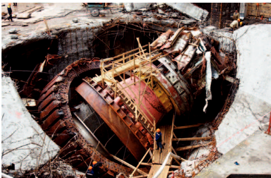
Figure 2. Part of the damage to the powerhouse after the 17 August 2009 accident. Unit 2 as seen on 3 September 2009 after dewatering.
