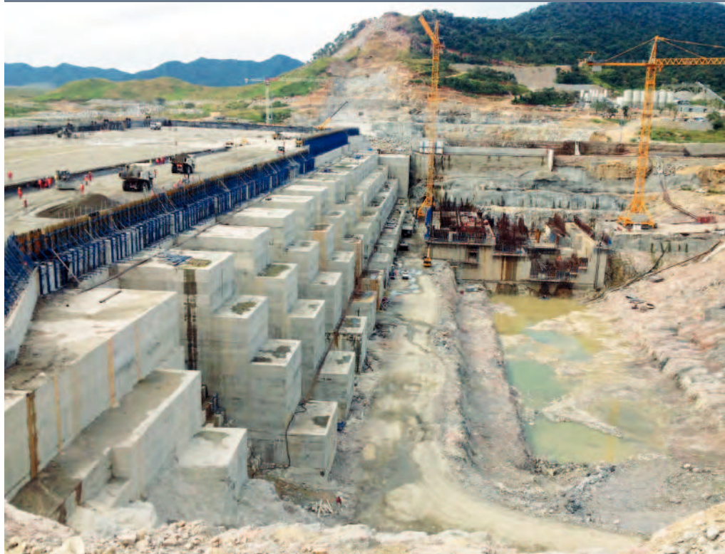
The Great Ethiopian Renaissance Dam project main dam view from the right abutment with the roller compacted concrete dam under construction, October 2014
