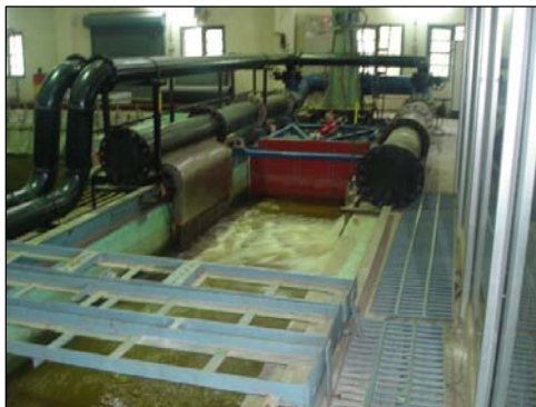
Fig. 8. Intake pipe exposed to wave and current
