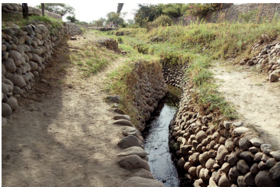
Figure 2. Cobble walls of Nazca canal downstream of filtration galleries. This irrigation structure is still in use
