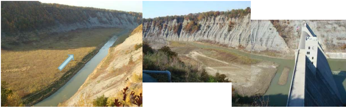
Figure 9 Reservoir sedimentation of Mount Morris dam in USACE Buffalo District (Left: Channel erosion, Right: Sediment deposited just upstream of dam is periodically dredged)
