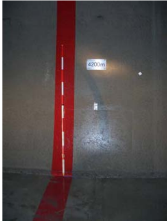
Status Inside Mibu River Bypass (Shortly after discharge on July 20)
