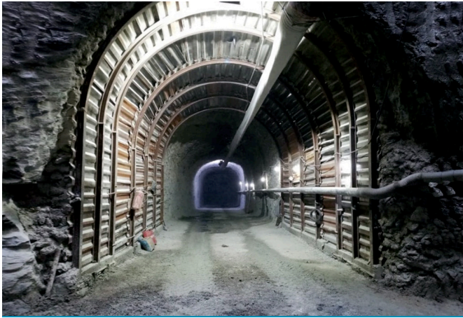
Figure 4 | SRO stormwater drainage tunnel under El Jadida road in western Casablanca.
