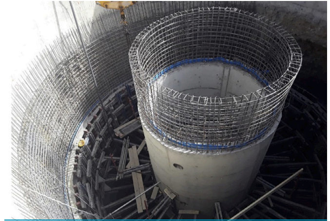
Figure 5 | A 4 m -diameter drainage well of the Hay Sadri neighborhood stormwater tunnel, part of the SRE system in eastern Casablanca.
