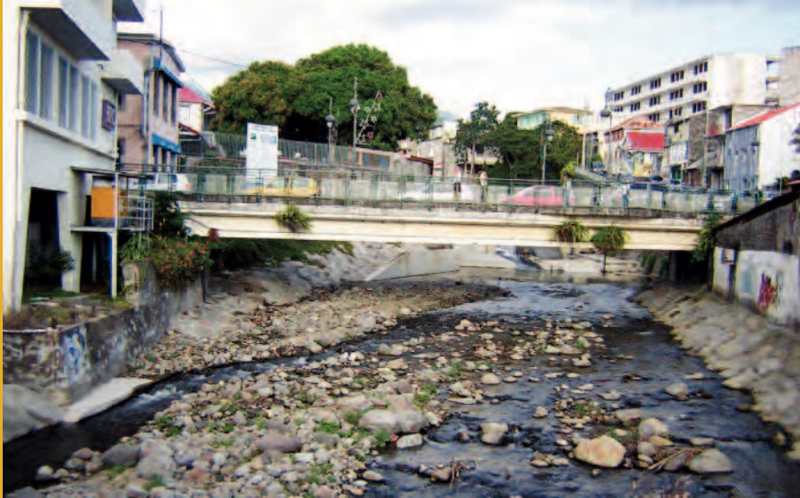
What will be the conveyance of the river during next flood?
