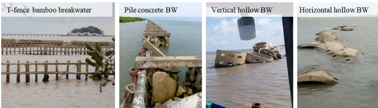
Figure 1: Some failure examples of breakwater in the MD (Source: images were provided by Ca Mau DARD).
