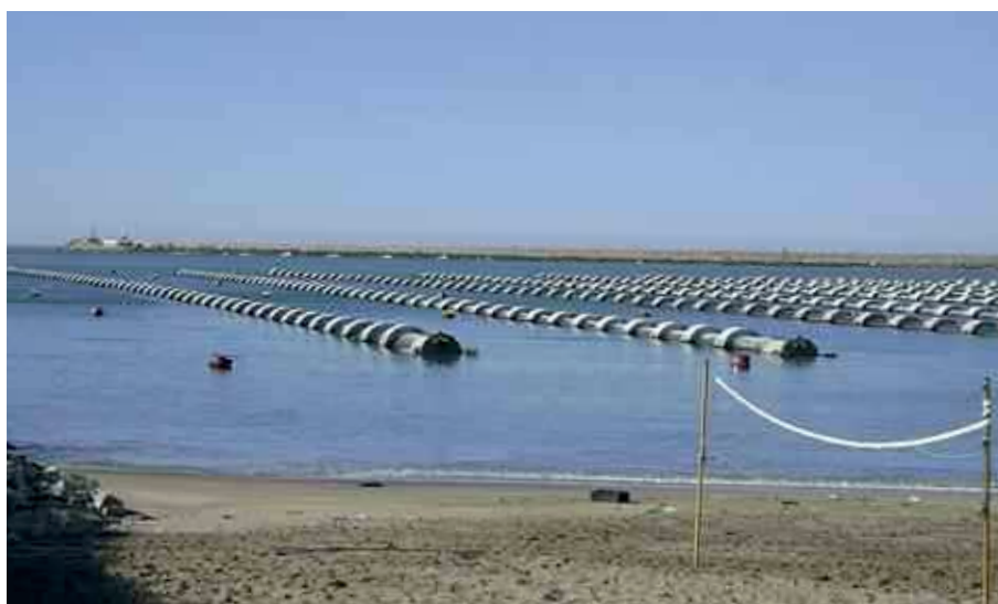
Figure 2. HDPE pipes comprising the manifold of the Mar del Plata (Argentina) sewerage outfall ready for installation. This photo was taken during a technical visit at the International Symposium on Outfall Systems in Mar del Plata Argentina, 2011
