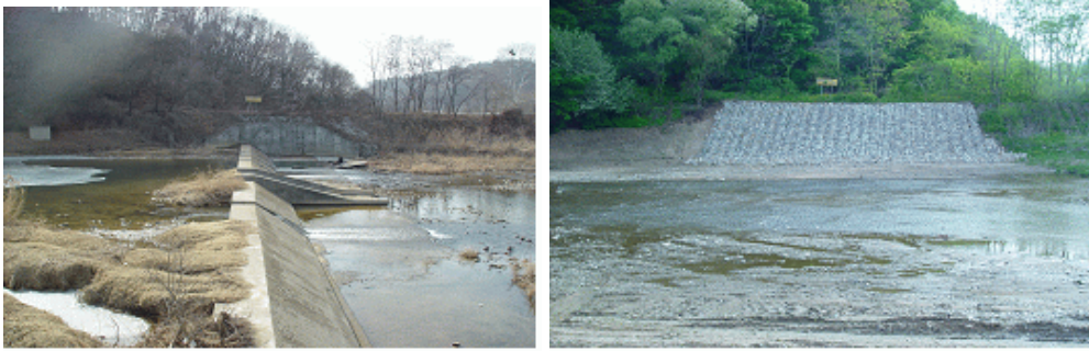
(Figure 6) The images of Gokreung weir 2 before (left) and after (right) the weir removal (left bank of the small dam)
