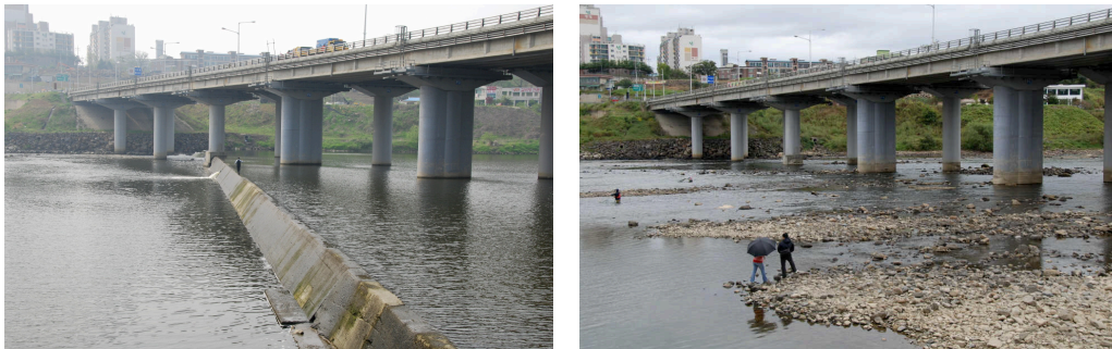
(Figure 7) The images of Gotan small dam before (left) and after (right) the dam removal (right bank of the small dam)
