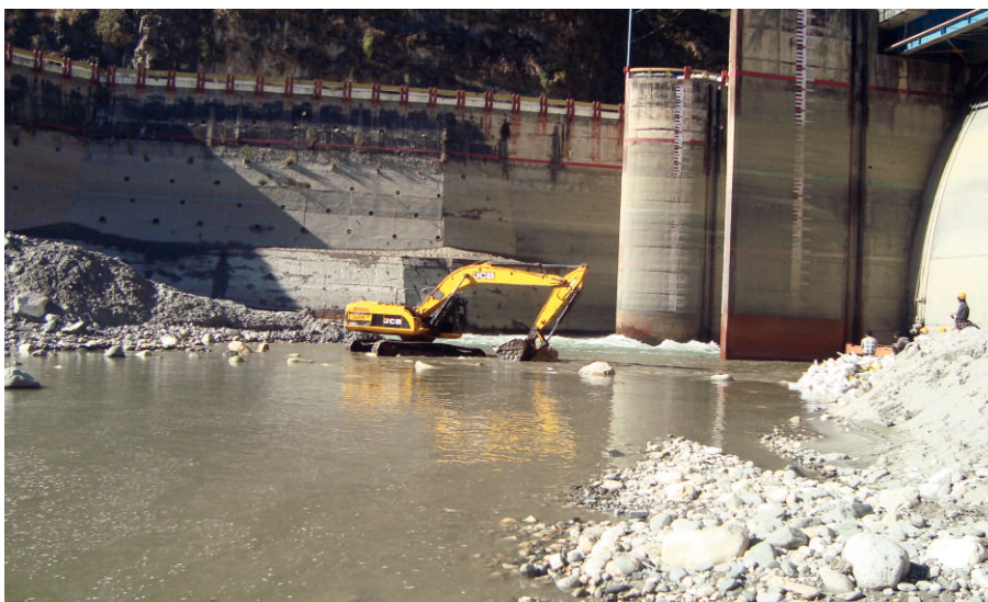
Figure 1. Sediment accumulation reduces storage volume and may interfere with the operation of dam outlet works. Removal of sediment by dredging or excavation (as shown in the photograph of the Maneri Bhalil Stage 1 dam during maintenance of the spillway.) may be needed to enable the dam to function.
