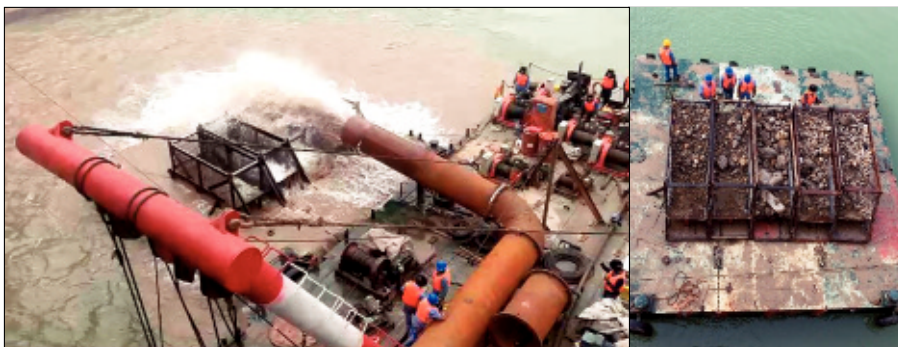
Figure 7. Dredging project of the tailrace canal of the Longkou reservoir in the Yellow River. The material diameter was 1 m.
