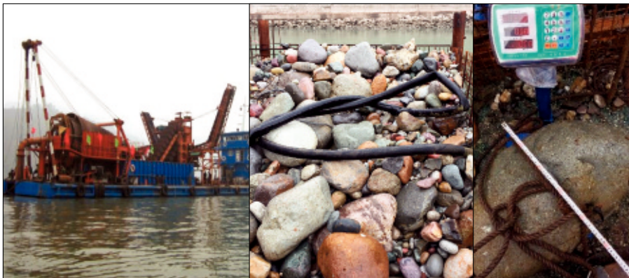
Figure 6. Jinping-II hydropower station in the Yalong Rive - Dredging operation showing the barge and removed material
