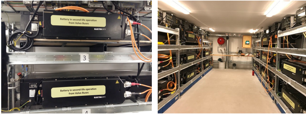
Figure 3.10: The second-life Li-ion batteries of Brf Viva.
