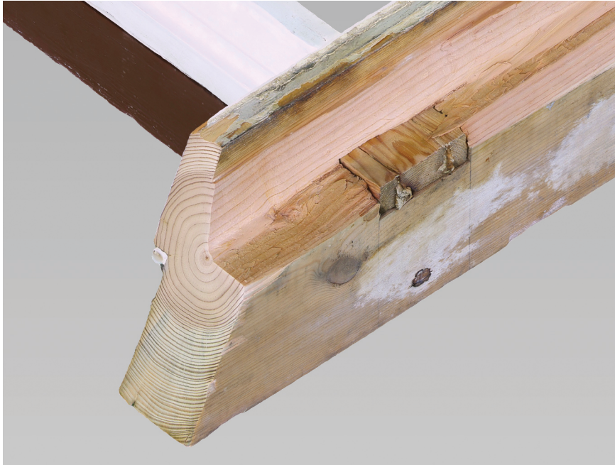
Figure 3.10. Completions , isometric view of three-dimensional geometry of salvaged window frame obtained with photogrammetry (cropped). Closed mesh model with image map.
