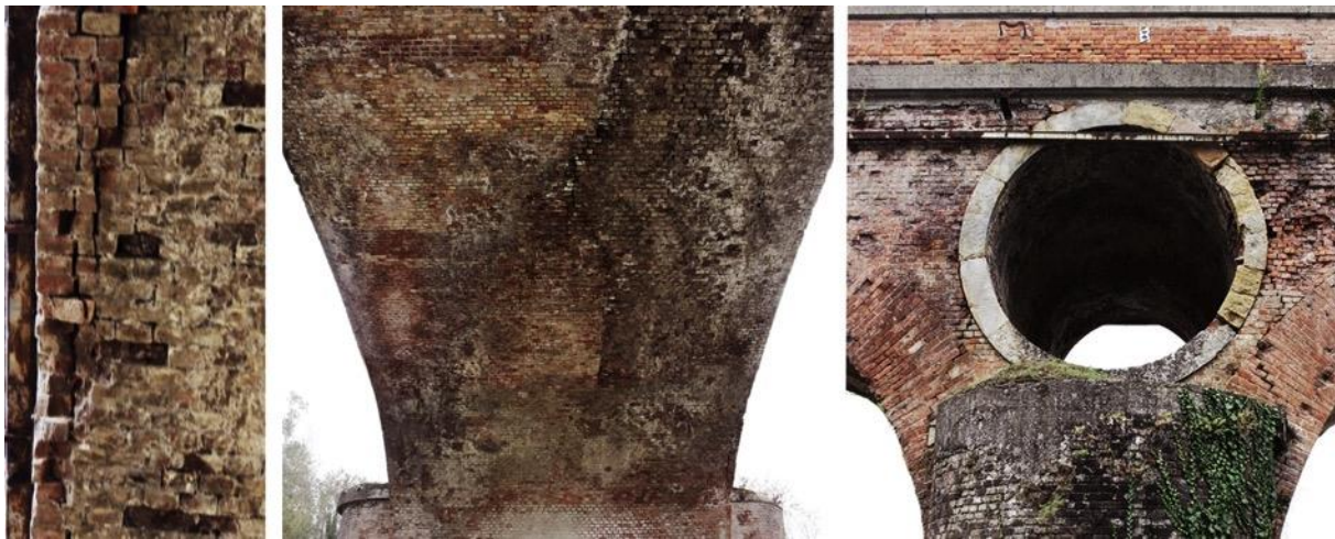
Figure 2: cracks caused by brickwork disposition, on the left. and structural fractures originated from differential deformations and settlements. In particular, in the center longitudinal crack on the intrados vault worsened by post-WWII reconstructions (span n.12) and, on the right, lateral cracks on the arch extrados (span n.17).
