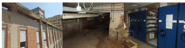
Fig. (25). Examples of degradation of concrete elements (left) and inadequate anchorage of plant systems (centre) and shelves (right) in [HB] building.
