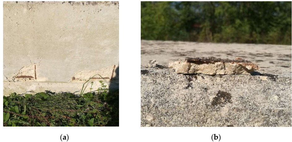
Figure 4. Spalling in column C after struck by hammer (a), detached cover due to hammer strike (b).
