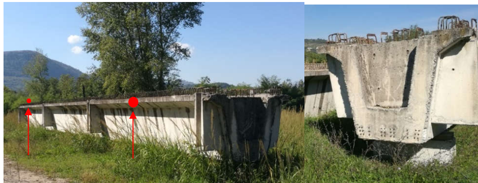
Figure 2. Prestressed RC omega-beam “B1”; red circles show the location of coring sites.
