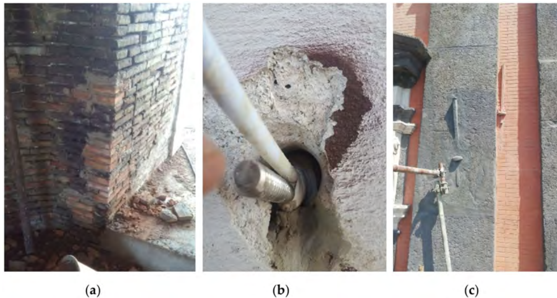
Figure 10. Masonry rebuilding (a); anchor with sock (b); restoration of oxidized metal elements (c).
