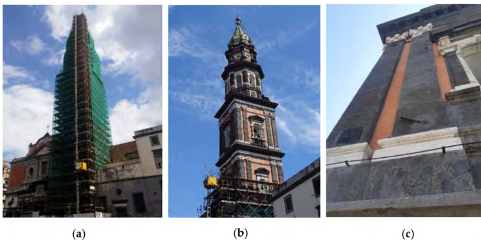
Figure 2. The bell tower with the scaffolding (a), during the dismantling of the scaffolding (b) and after completion of works (c).
