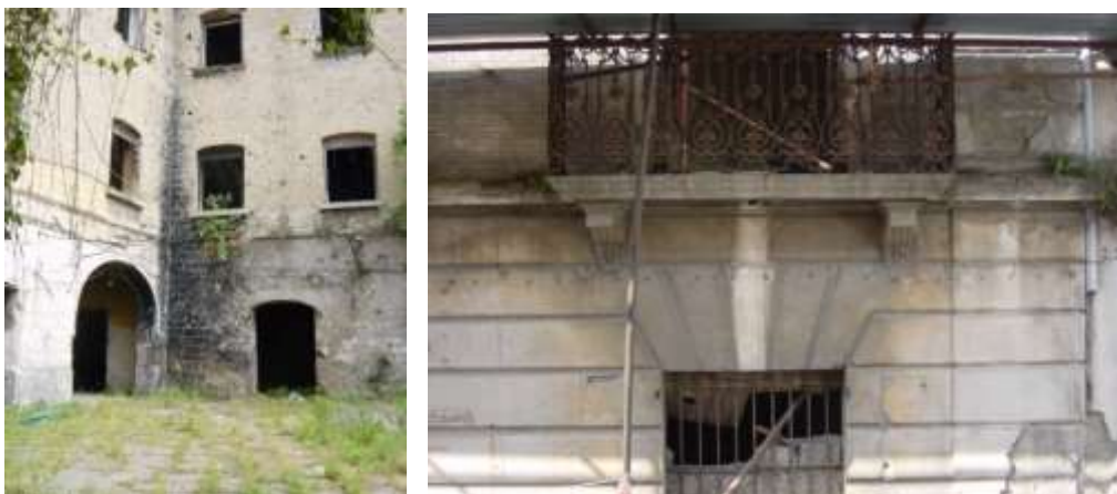
Figure 4 (a) and (b). The current deterioration of the building
