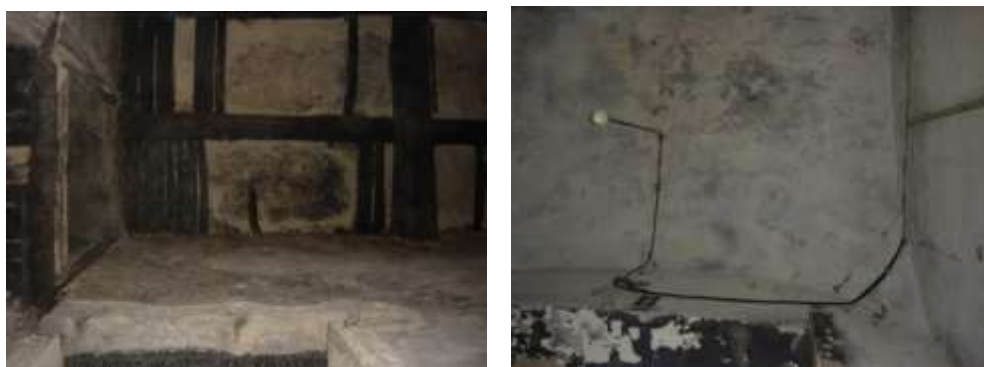
Figure 13 (a) and (b). Degraded plaster and false ceiling
