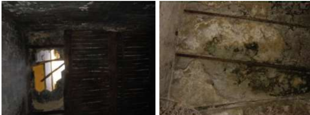
Figure 12 (a). Collapsed wooden floor; (b) Rusty iron
