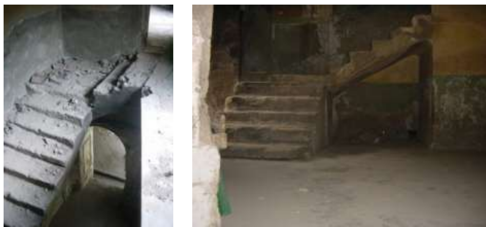
Figure 14 (a) and (b). Collapsed stairs
