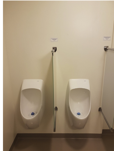
Fig. 1. Waterless urinals. A waterless urinal can reduce the use of water significantly and indirectly reduce CO 2 emissions.
