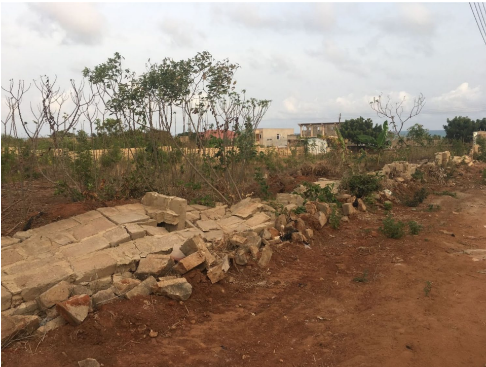
Figure 2. A fence wall pulled down by Landguards. Source: Fieldwork photo, 2018 (By Divine Asafo)
