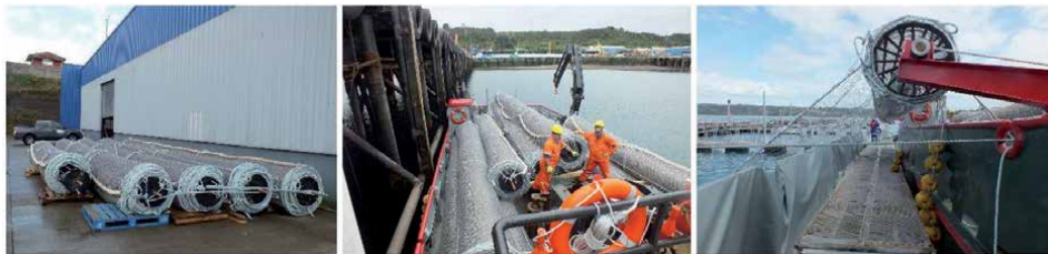
Figure 7. Installations in South America - Total 112'000 sqm.
