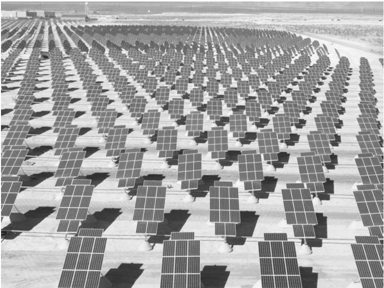
FIGURE 4.5 Nellis Air Force Base Solar Power Farm. This photograph shows a solar farm made up of individual sun-tracking collectors, each comprising twelve individual PV panels. Space for access between collector units and for support buildings such as those seen in the background here reduce the amount of solar power that can be captured within a given solar power farm footprint area.
