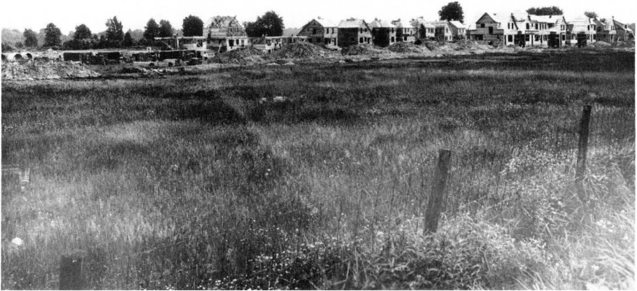
Figure 13. This view of the early stage of Ford Homes construction indicates the orderly succession of specialized crews, who were assigned to excavate, lay foundations, frame, and finish rows of houses. Horse-drawn, narrow-gauge railway cars brought materials, precut and assembled, from on-site shops to the building site.
