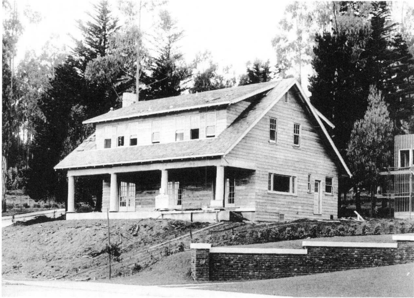
Figure 30. 185 Westwood, Westwood Park, under construction. Hans Nelson, builder, and Charles Strothoff, architect, were among the many builders and architects working at Westwood Park. They collaborated on the construction of this house before Baldwin and Howell hired them to design and build Westwood Highlands.
