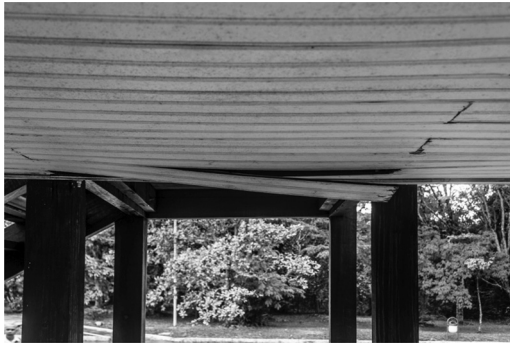
Figure 8. Ceiling on the ground floor of the Catetinho showing deterioration. P.P. Palazzo, 2017.
