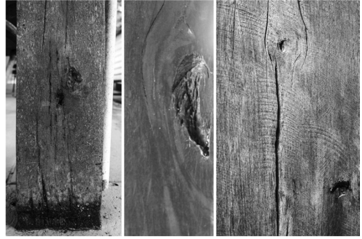
Figure 9. Posts showing damage by rot, loss of supporting section creating a habitat for insects and arachnids, and cracking due to buckling. M.M. Mennucci, 2017.
