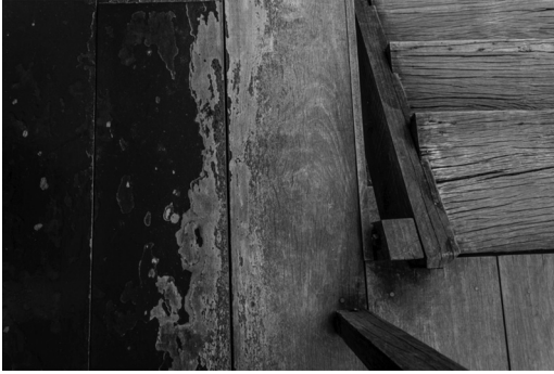
Figure 7. Veranda floor and stairs showing deteriorated paint coat in exposed areas. M.M. Mennucci, 2017.
