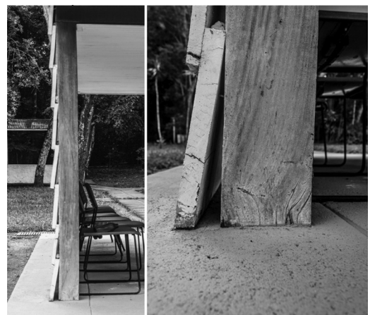
Figure 5. Side view and detail of clapboard bracing at the Catetinho. M.M. Mennucci, 2017.
