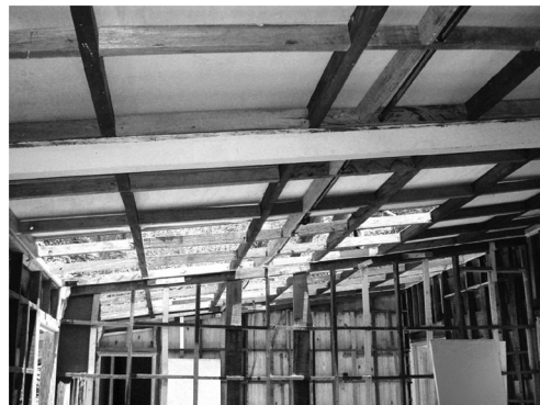
Figure 4. Replacement of the interior sheathing in progress, showing roof structure, first half of February, 2012. Federal District Historic Preservation Office (Supac) digital archive.
