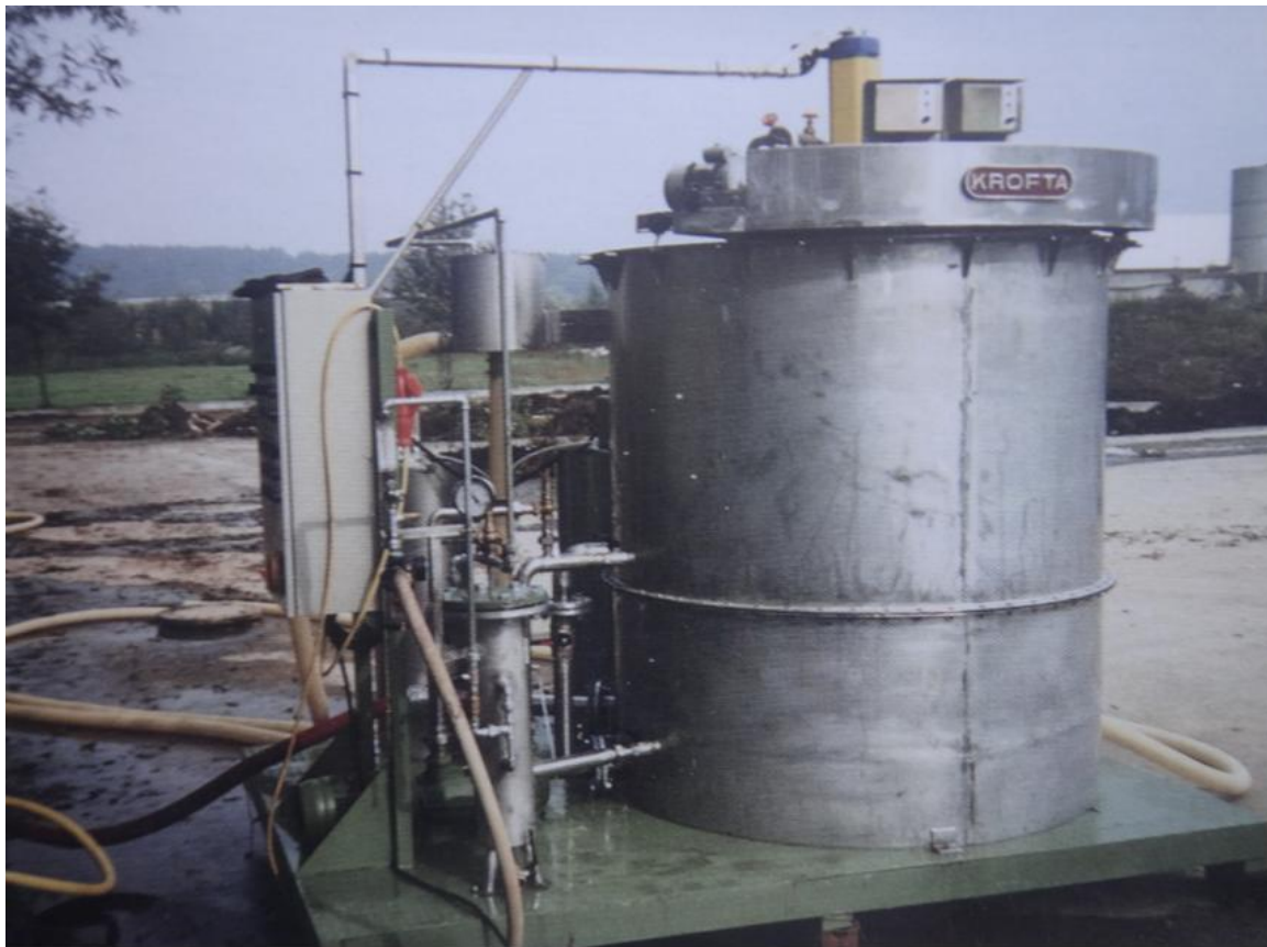
Figure 4. A Picture of Mobile Sandfloat DAFF Type 8 Package Plant
