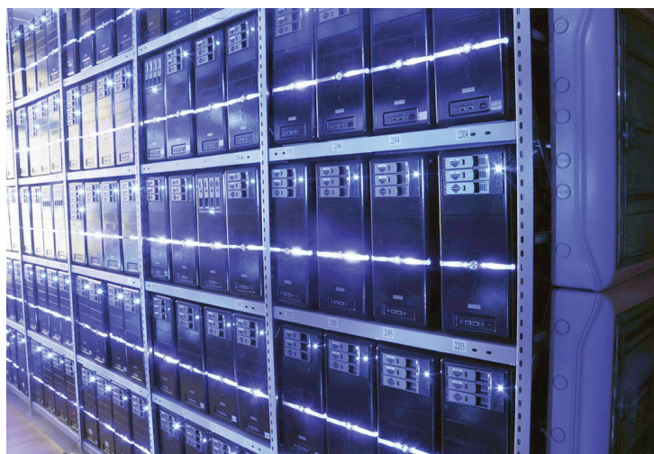
Servers in a data center. The “cloud” is always just somebody else’s hard drive Photograph by Baltic Servers
