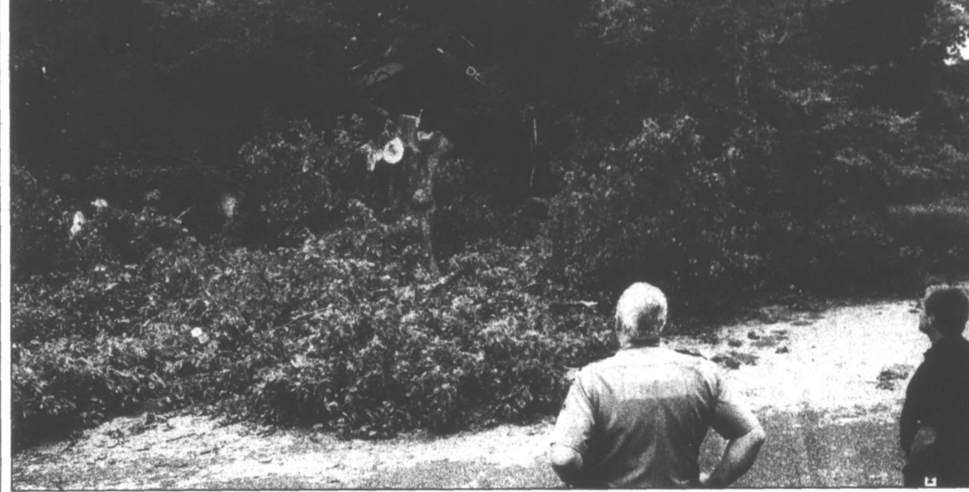
JOHN WRIGHT/Ledger & Times City of Murray Code Enforcement Officer Tim Fortner, left, and city Building Official Keith Miller survey the demolition of an abandoned house Wednesday morning along North Cherry Street.
