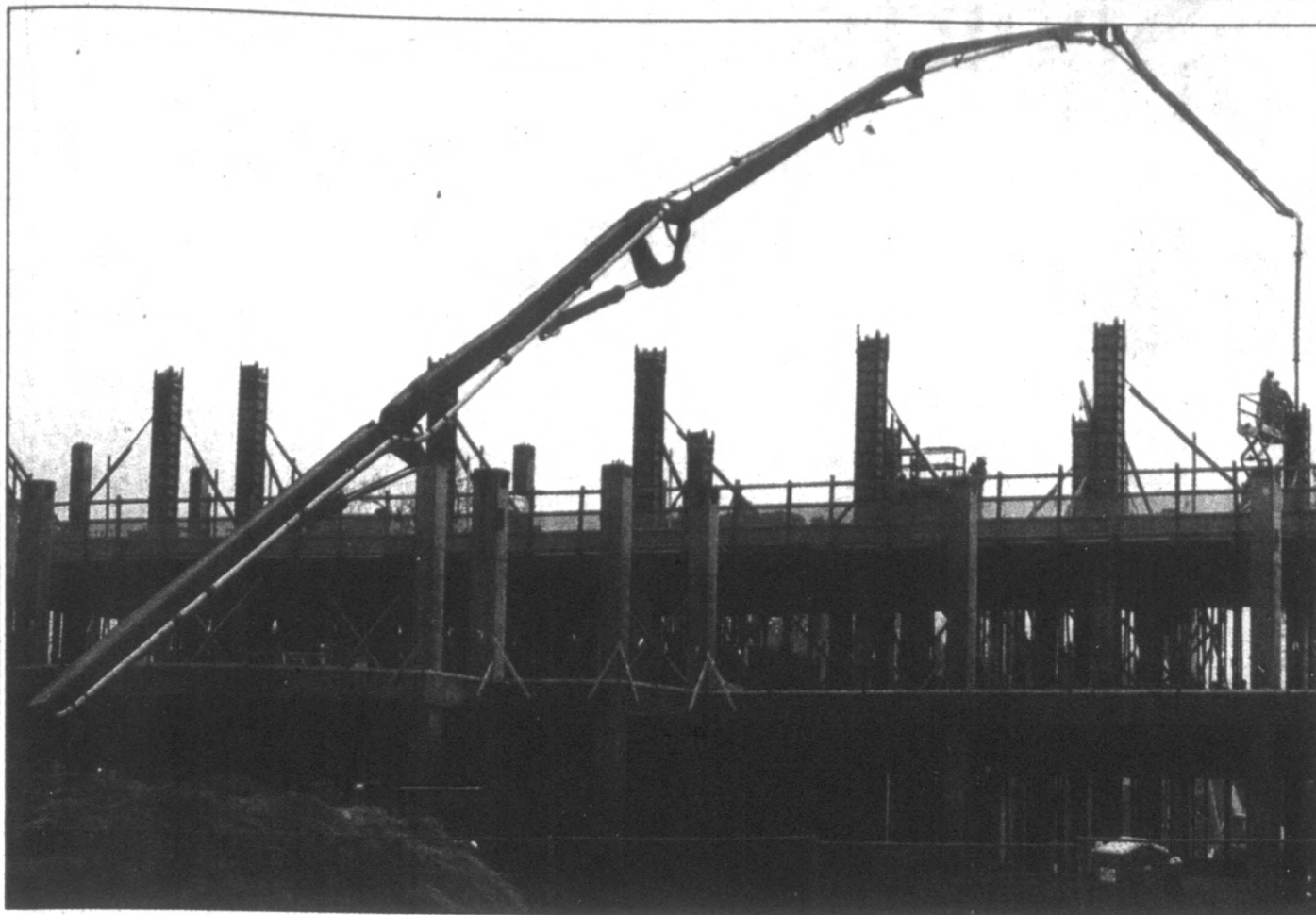
GETTING IT THERE ... ONE WAY OR ANOTHER: A concrete pumping machine forms a large arch as it stretches to provide cement to an area of the Engineering & Physics Building under construction along North 16th Street on the Murray State University campus.
