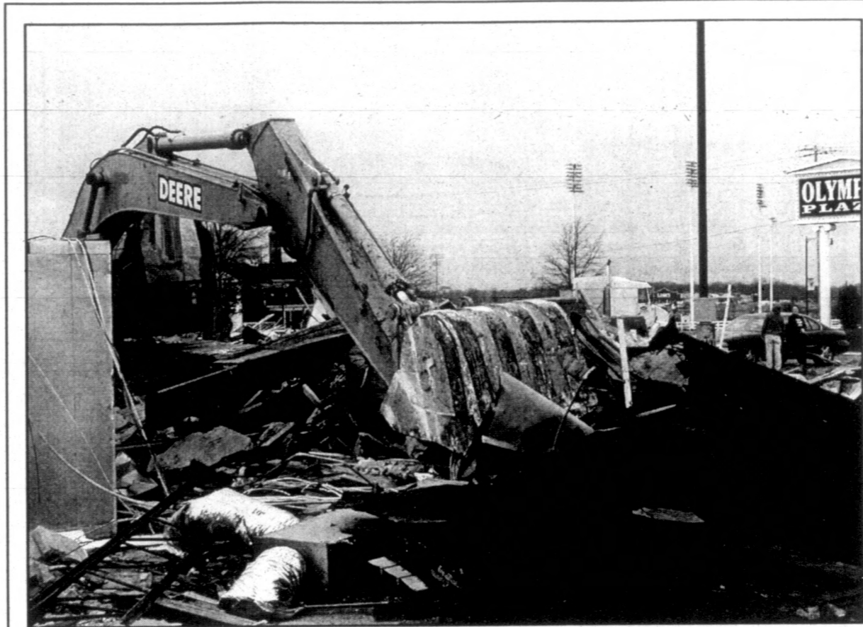
JOHN WRIGHT/Ledger & Times photo Johnny Rains of Murray's Bogard Trucking & Excavation Company sits at the controls of a track hoe machine as it demolishes the building that once housed a Subway/Baskin Robbins Ice Cream shop at the Olympic Plaza on North 12th Street. A company spokesman said the demolition was performed in order to produce more parking space at the shopping center.
