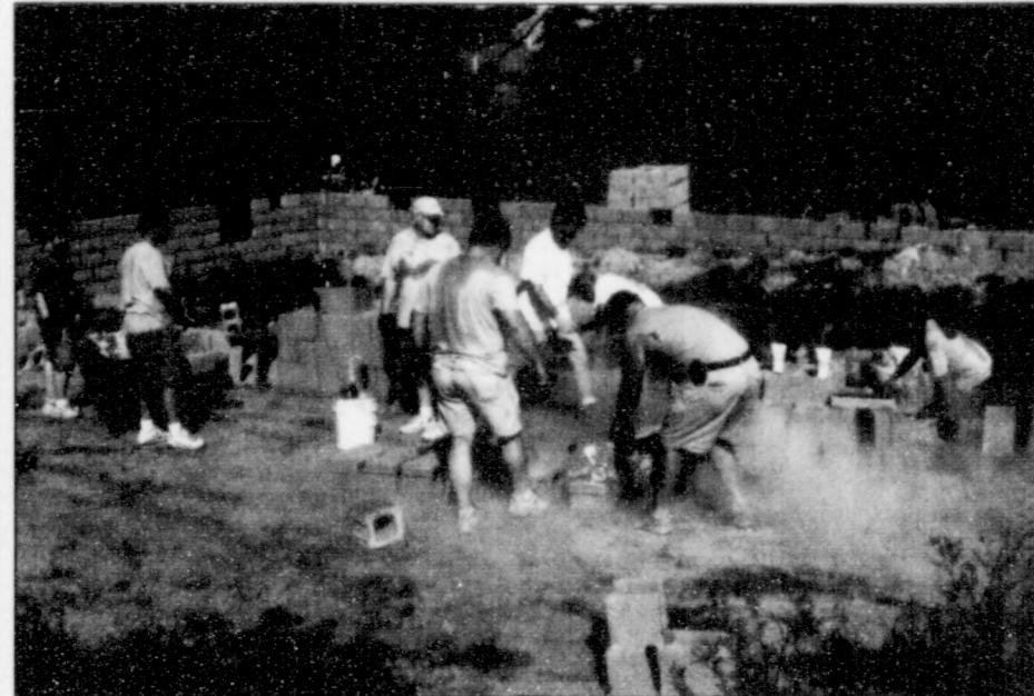
Photo provided Pictured are a group of volunteers working on the foundation of the new Habitat for Humanity house.
