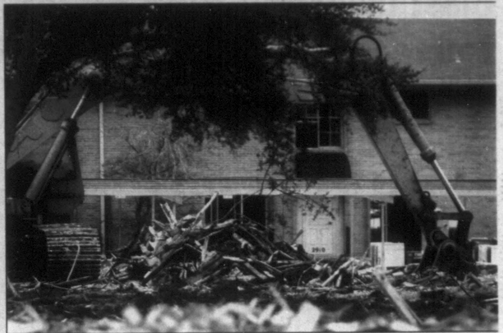
Demolition of an apartment housing area is seen near the SMU campus in Dallas on Thursday. The area is reported to be part of the proposed location for the George W. Bush Presidential Library.
