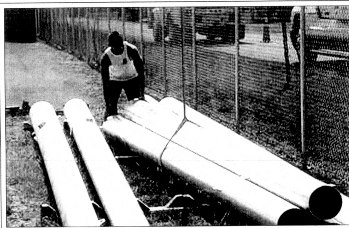
LET THERE BE LIGHTS...Murray High School graduate Gary Crass, a place-kicker for the Tiger football team and a preferred walk-on at Murray State University, helps Murray Electric System unload the lights and poles for the soccer field at MHS' Mallary France Athletic Complex Wednesday.
