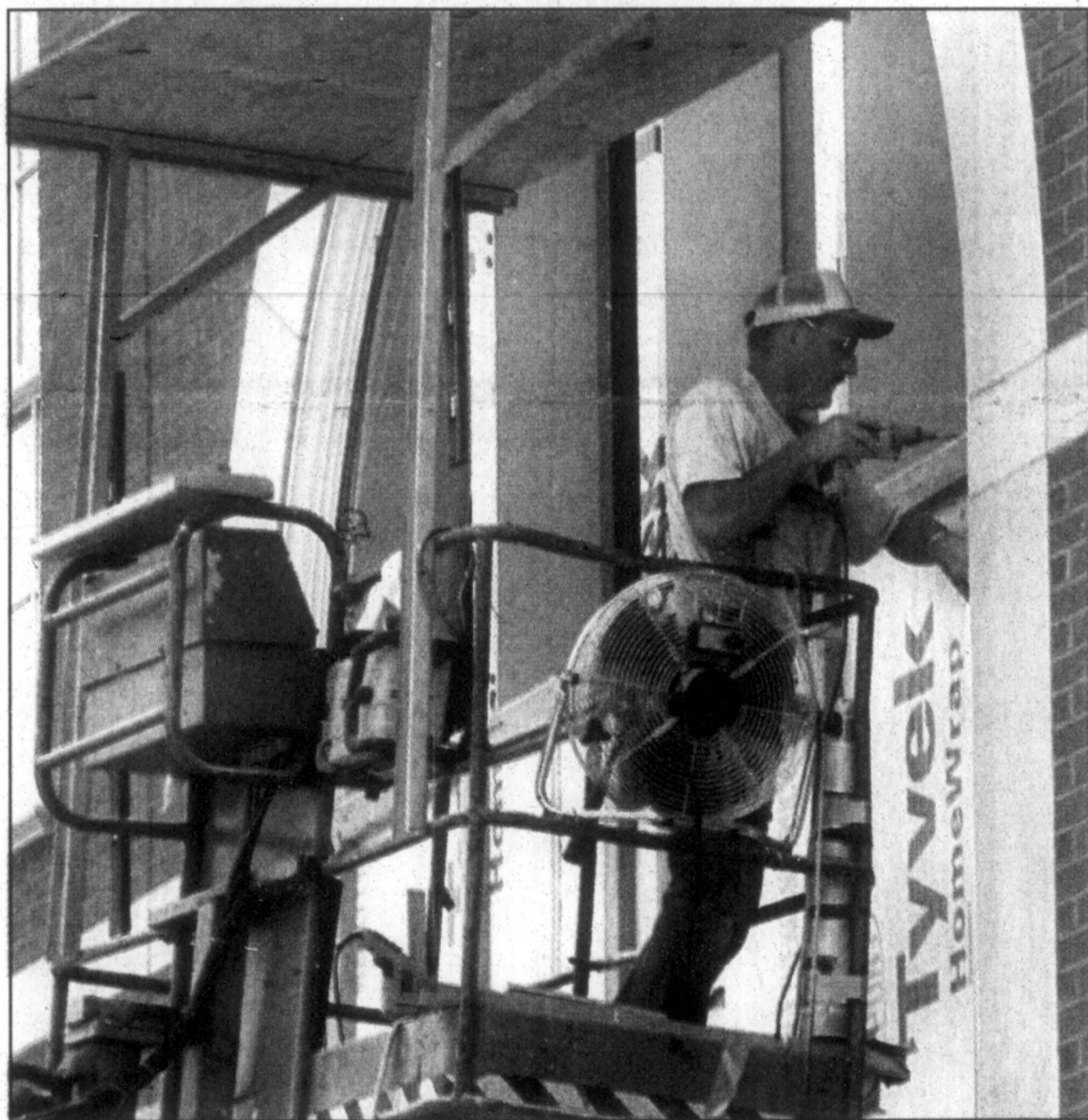
BERNARD KANE/Ledger & Times Photo HERE'S THE DRILL ... Charlie Hartle tries to keep his cool with a sunroof and a fan as he installs window frames on the new addition to the Murray State University education building one afternoon.
