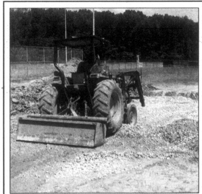
BERNARD KANE/Ledger & Times Photo MAKING THE GRADE ... Murray Calloway County Parks employee Robert Young grades what will be the foundation for the new pavilion between the baseball fields at the Hohman Fields complex Tuesday. The construction of the building will begin Monday.
