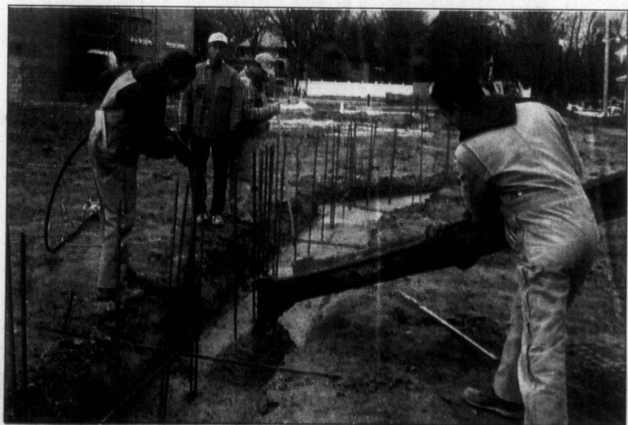
Construction workers pour a 33-inch-wide earthquake-proof footing for the new Murray-Calloway County Hospital fitness center on Wednesday.
