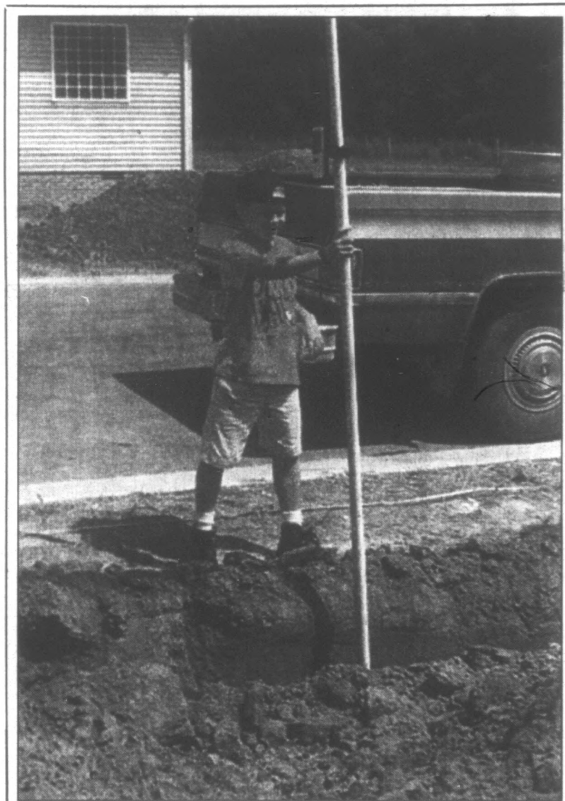
EASY WORK: Stephen Hill, 8, helps with the construction of a sewer main by shooting the elevation for his dad Roy's Backhoe Service in the proposed annexation area on Stairview Drive Monday.
