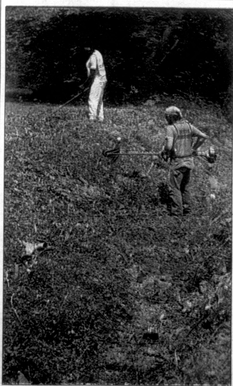
FINISHING TOUCHES: Murray Street Department crews on Wednesday remove the last of the weeds that had covered a drainage ditch on 13th Street. The crews also cut brush and small limbs as part of the cleanup.
