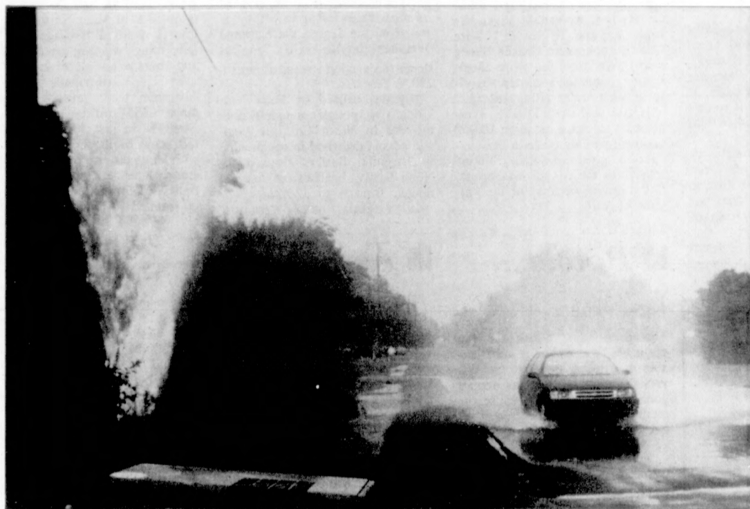
OOPS: Workers from Network Communications and Paging Company were digging a ditch for cable lines Monday off 18th Street, when they accidentally hit a water main. Water from the line shot an estimated 50 feet in the air.
