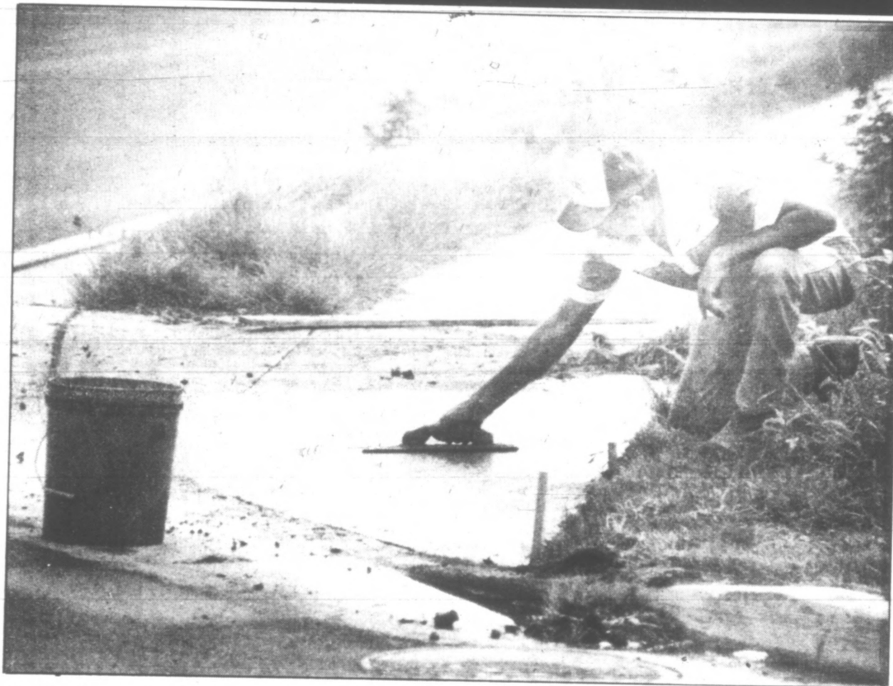
Construction worker Phil Parrish stretches with a trowel as he smooths some freshly-poured concrete at a curb on Glendale Road. Parrish, a Cadiz resident, is employed by Wilkins Construction Co. of Paducah.
