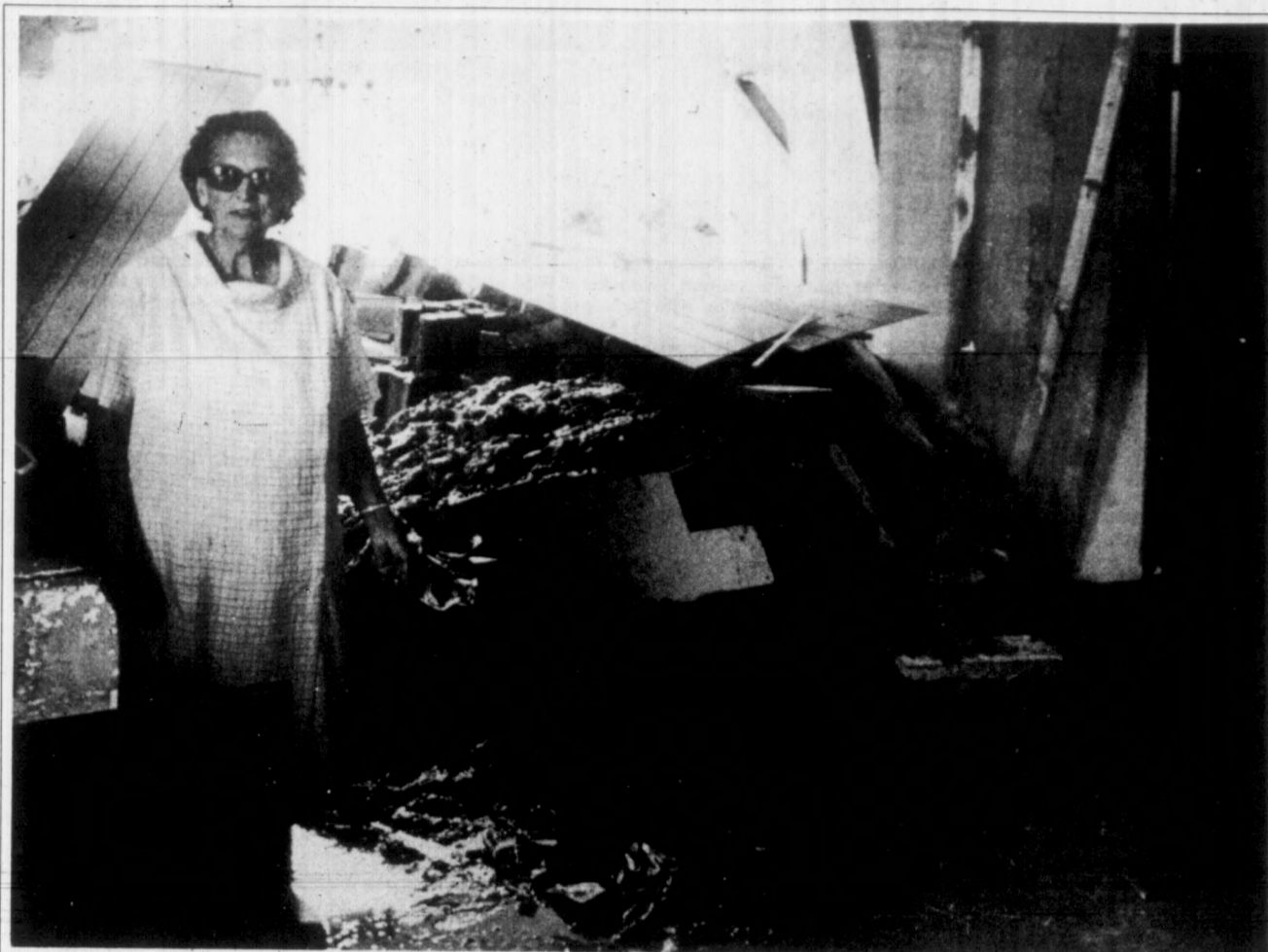
RAIN DAMAGE — Several reports of damage resulting from Tuesday morning's extremely heavy downpour were cited, but, standing in what was her kitchen, Mrs. Eulala Mardis, Route 3, gives a personal testimony to the amount of destruction left by the rainstorms. Friends, neighbors, the sheriff's department, and
