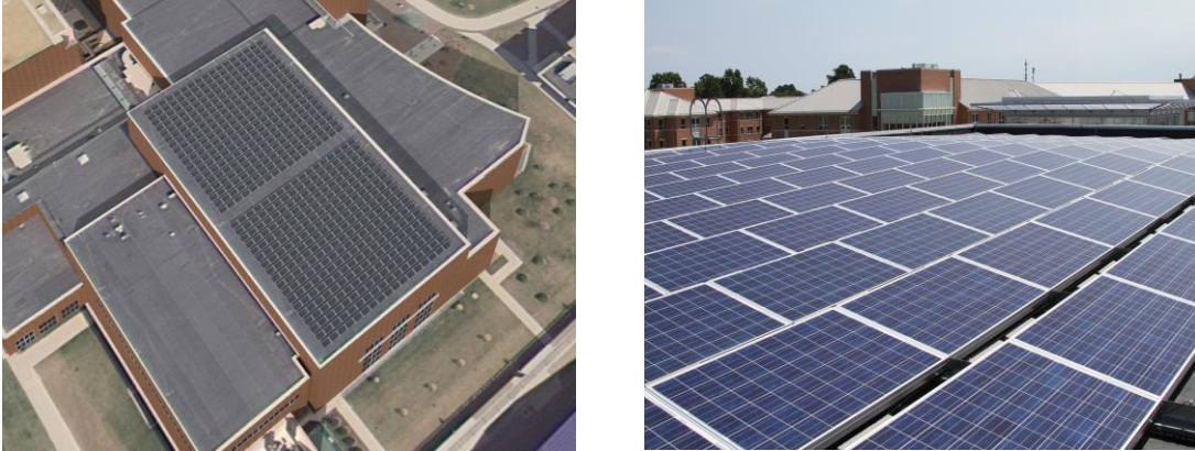
Exhibit 3. Views of the photovoltaic panels on the roof of Student Rec Centre at ODU.
