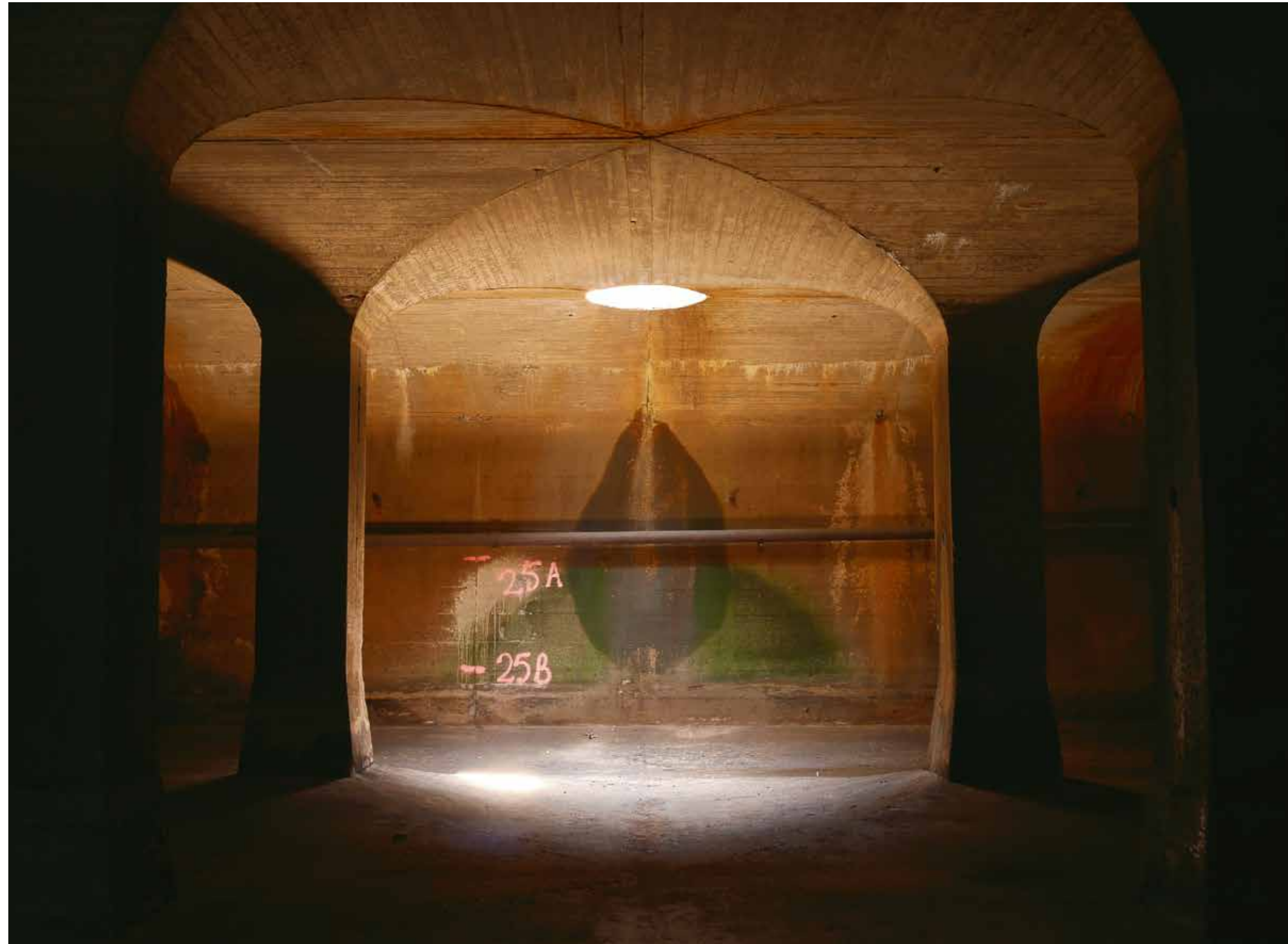
At the McMillan Slow Sand Filtration site, the barrel-vaulted ceilings culminate in a 3-foot diameter manhole
