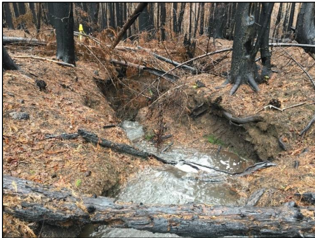
Figure 9. View downstream from within the tributary to SWP showing channel incision and bank erosion in Dec-20.
